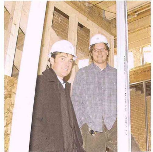
Greg Lobdell and Jon Carlson in the interior of the former Mayer-Schairer building.
